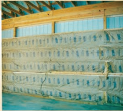
R-19 Wall insulation Must be covered with drywall or liner panel
